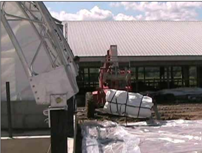
Cover is set into position next to the frame. Customer-supplied plastic film is shown on the site to protect the cover and to keep it clean during preparation.
