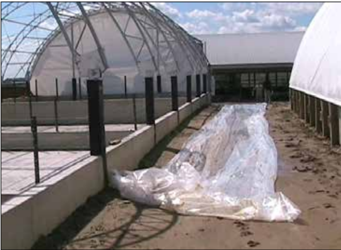
Photo above shows plastic (customer-supplied) on the ground to protect cover during preparation and installation.
