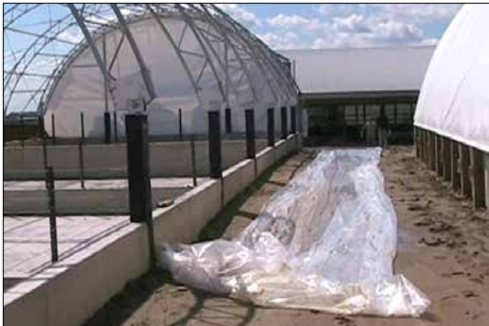
Photo shows plastic (customer-supplied) on ground to protect cover during preparation and installation.
