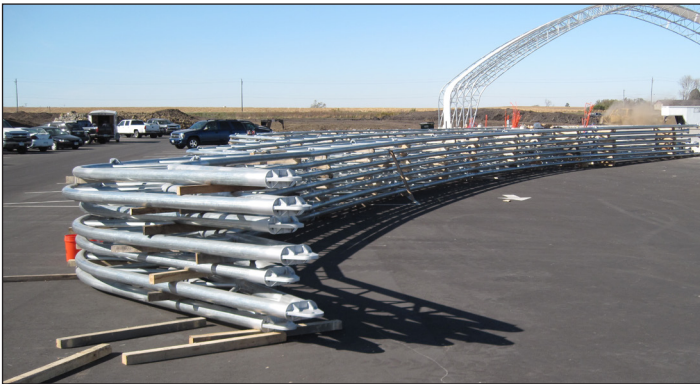
Photo above shows a stack of assembled trusses ready to lift and set in position on the base plates attached to the foundation.
