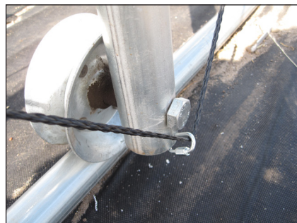
Photo to the right shows rope threaded through a quick link at the end of the rafter.
