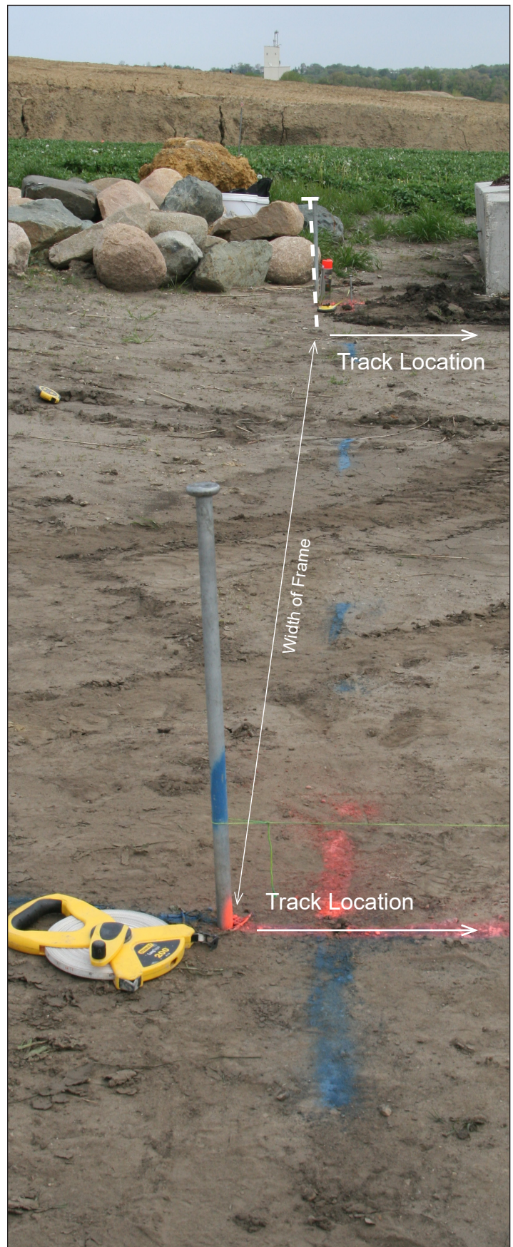
Photo shows stakes at the width of the frame and at the beginning of the track positions.
